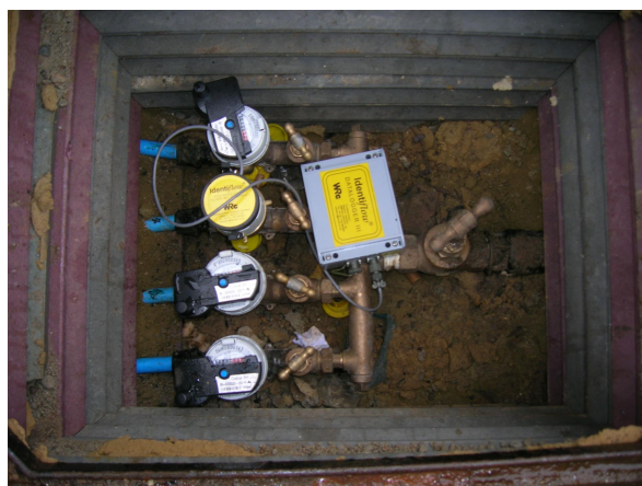
Identiflow® in action – monitoring flow into a flat
